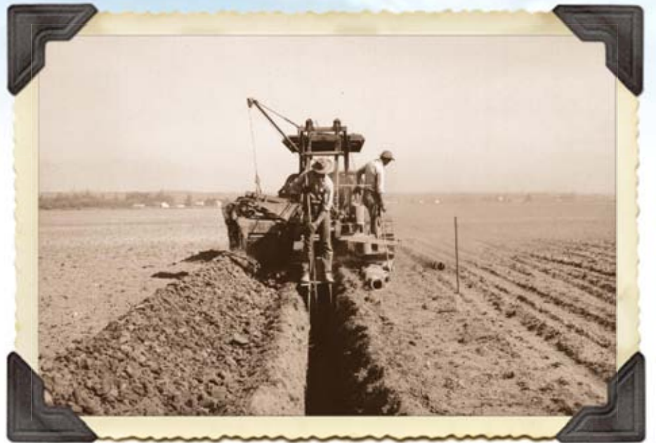
Underground tile lines being installed to increase drainage in a crop field. (Photo by A.F. Harms, 1951, Birger Johnson Farm).
